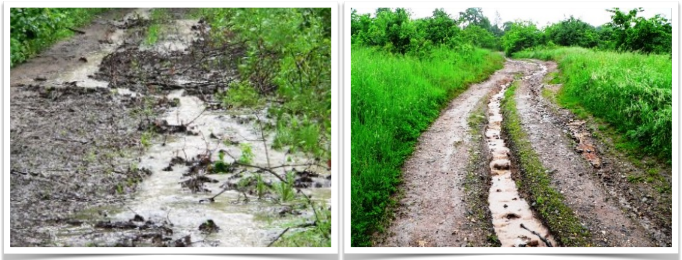
After the flood, waters carried the sediment away, depositing it downstream, eroding the road.
