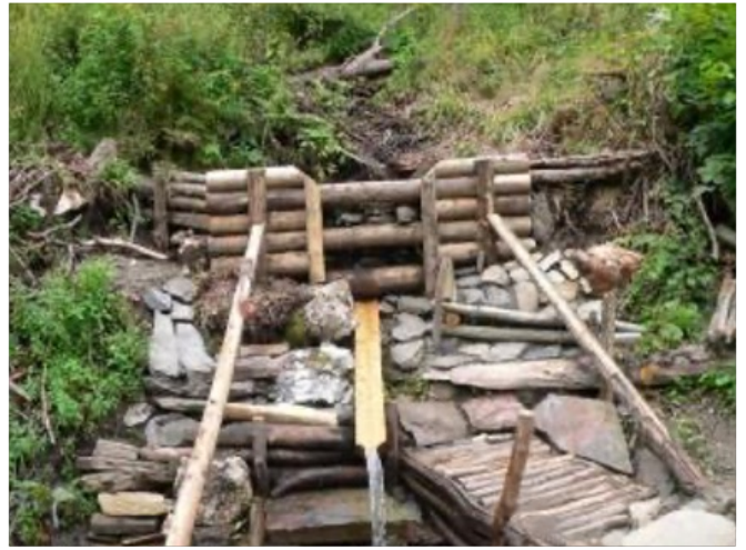
Elaborate check dam.
